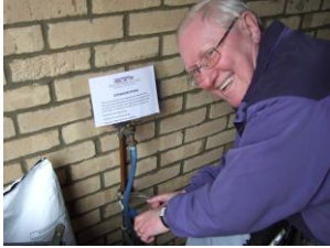
David gets to work fixing the pipe burst
