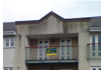
One of the stained areas: before and after cleaning.
