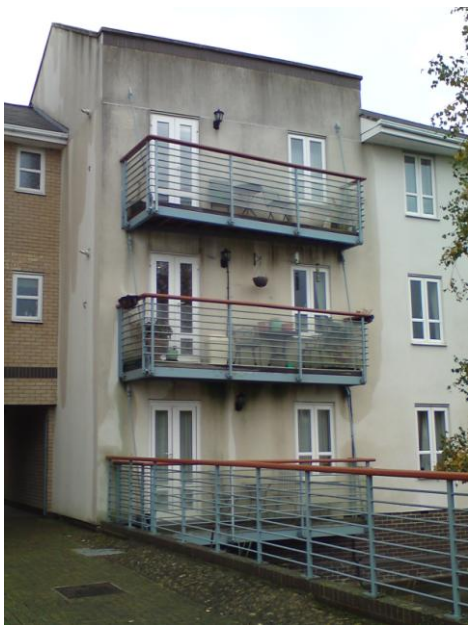
Example of wall staining around properties 9, 10 and 11.
